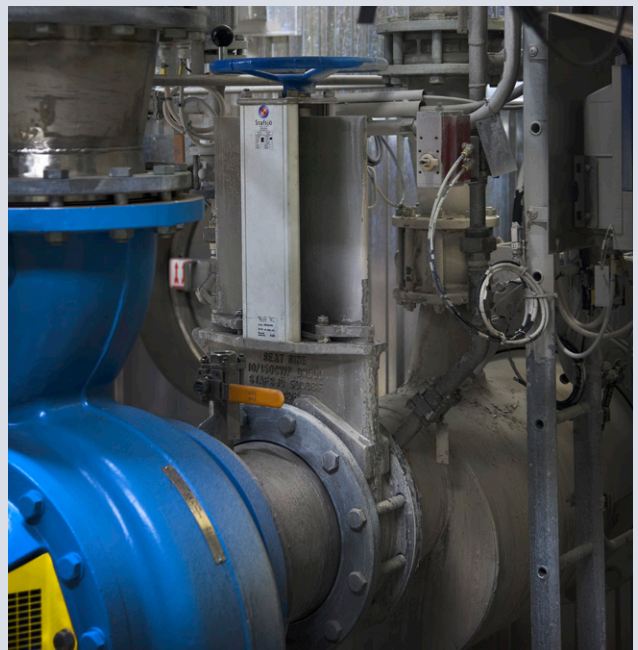
DN 300 / 12" Stafsjö MV installed on pump suction side.
