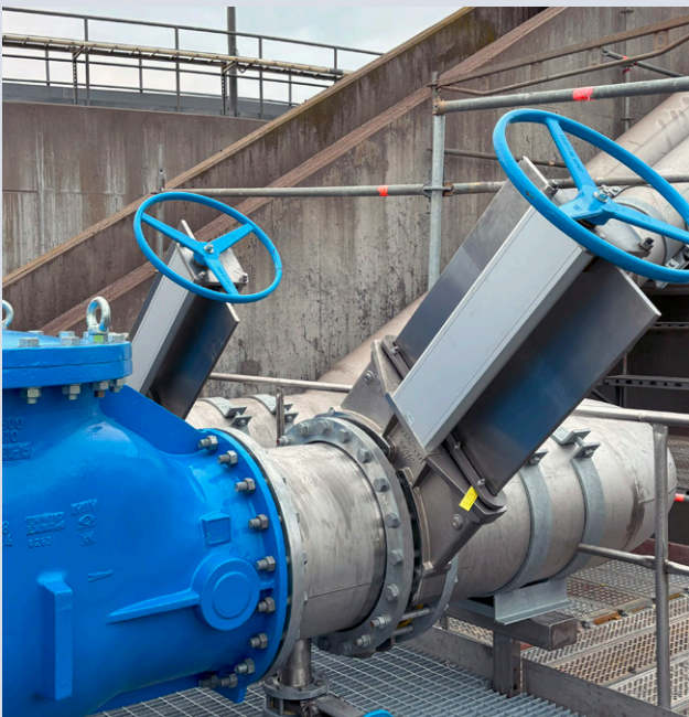
DN 600 / 24" Stafsjö MV serves as maintenance block for the check valve.
